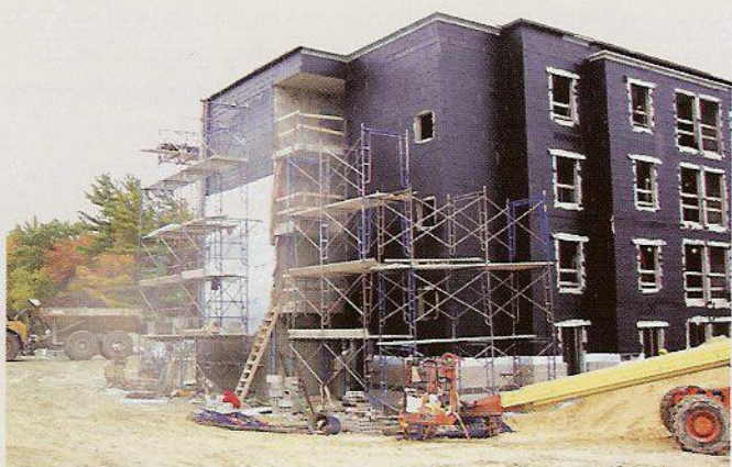
Installation of air barrier in progress at the dormitory buildings at the University of Massachusetts-Dartmouth Photo courtesy of ADD Inc.
